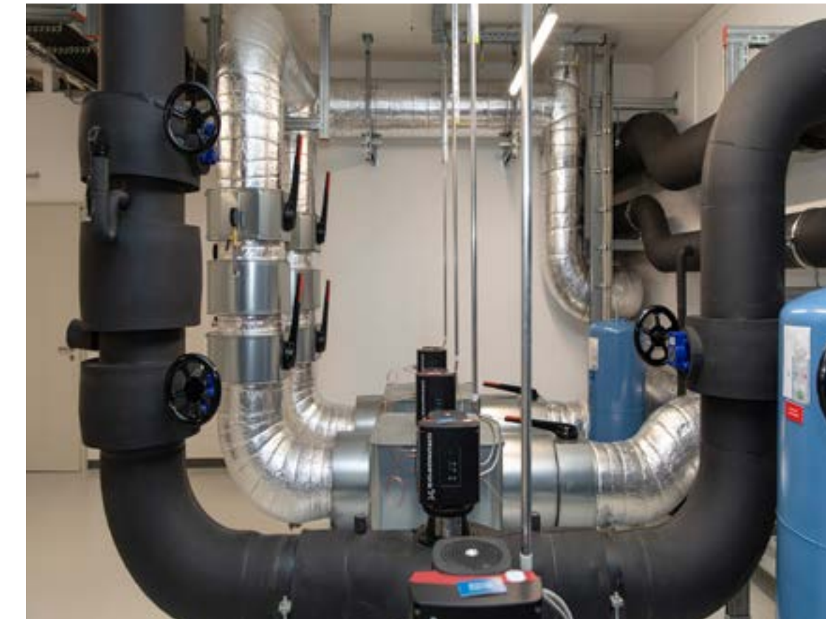
Pump house at company headquarters in Oberschleissheim
